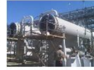
Liquid Natural Gas Filtration System
